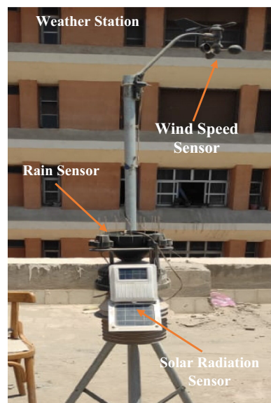
Fig. 3 A photograph of the weather station.
